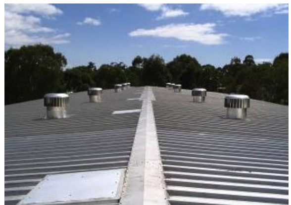
ecopower installation in Alexandra Hills State high school
