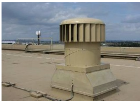
Ecopower installation on Mecure Hotel, Sydney Airport
